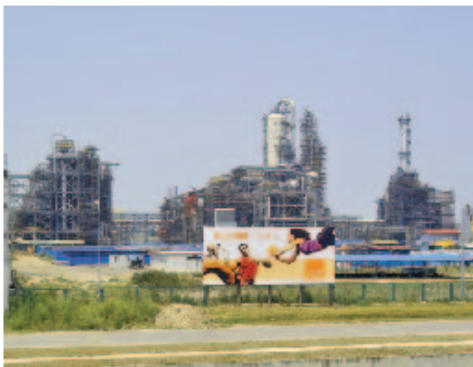
BASF PolyTHF (polytetrahydrofuran) plant at the integrated production site at the Shanghai Chemical Industrial Park (SCIP) in Caojing, Shanghai
